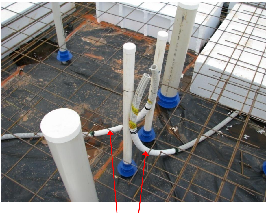
Above: Conduits resting on the moisture membrane have been protected by wrapping the end of each conduit.
